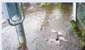
Water may gush out from the drainage channels. (Shinkawa area)
